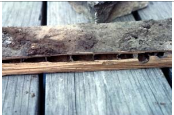
Damage caused by carpenter bee
